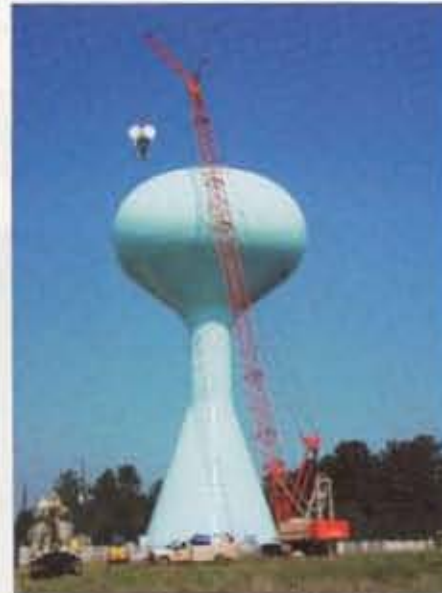
Boyer Inc's 100-ton crane placing a fully dressed antenna pod atop a water tower in Houston.
