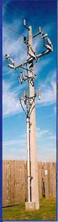
Customer owned switch pole
