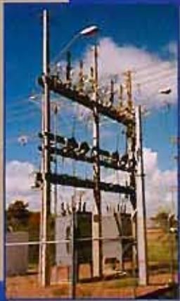
Substation area lighting and power distribution
